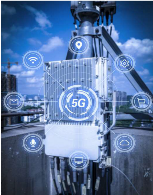
» 5G smart cellular network antenna base station.
