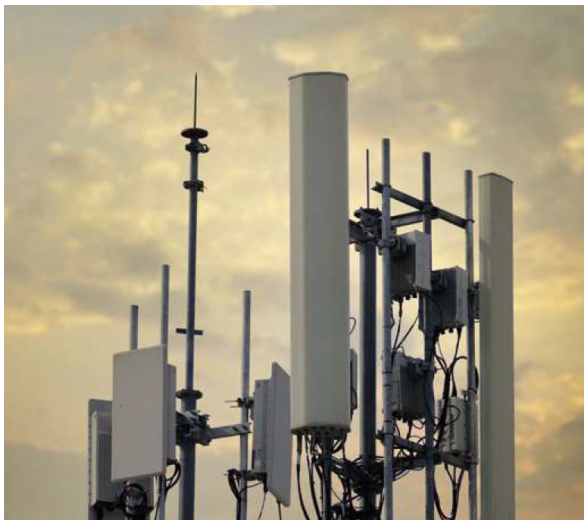
» 4G and 5G wireless communication tower.
